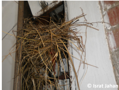
Image 17. Common Myna nest in electrical box
